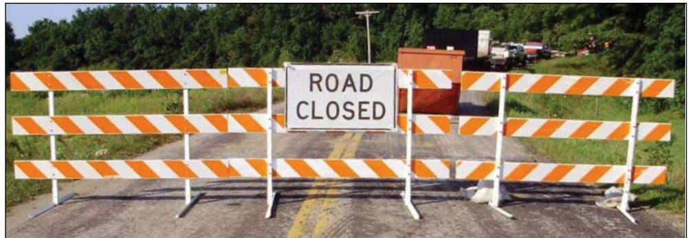
One Type III barricade should be used for every 8 feet of roadway with an unobstructed "Road Closed" sign attached to the forward most barricade.
