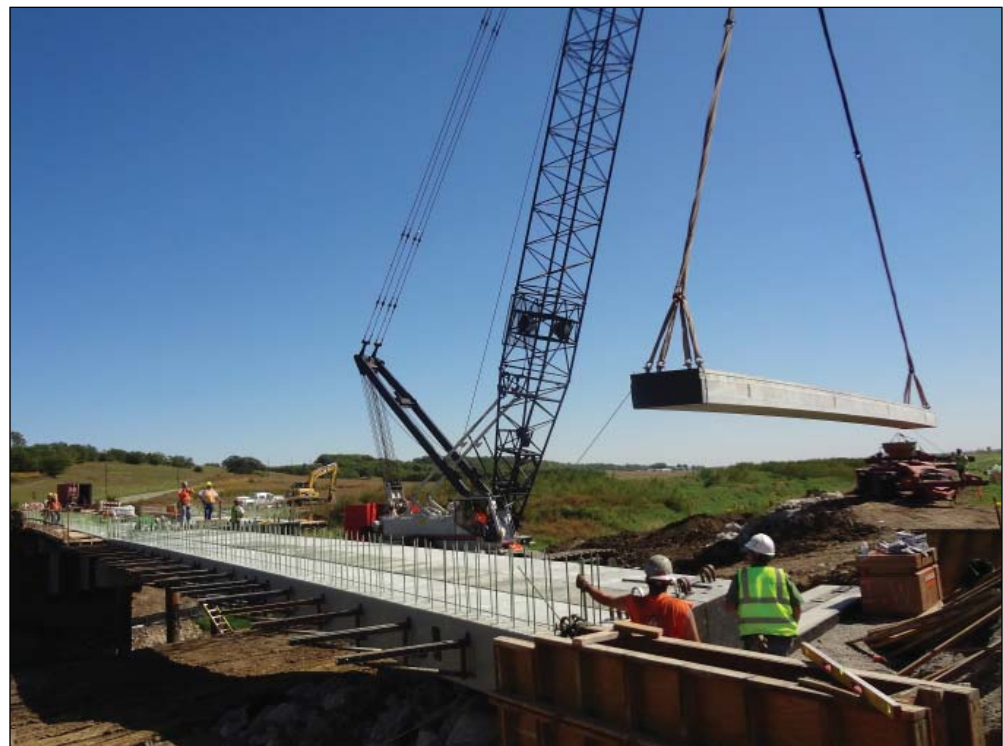
Clarkson Construction Co. sets 80 foot adjacent box beam girders for Bridge B0088 on US Route 59 in Holt County.
