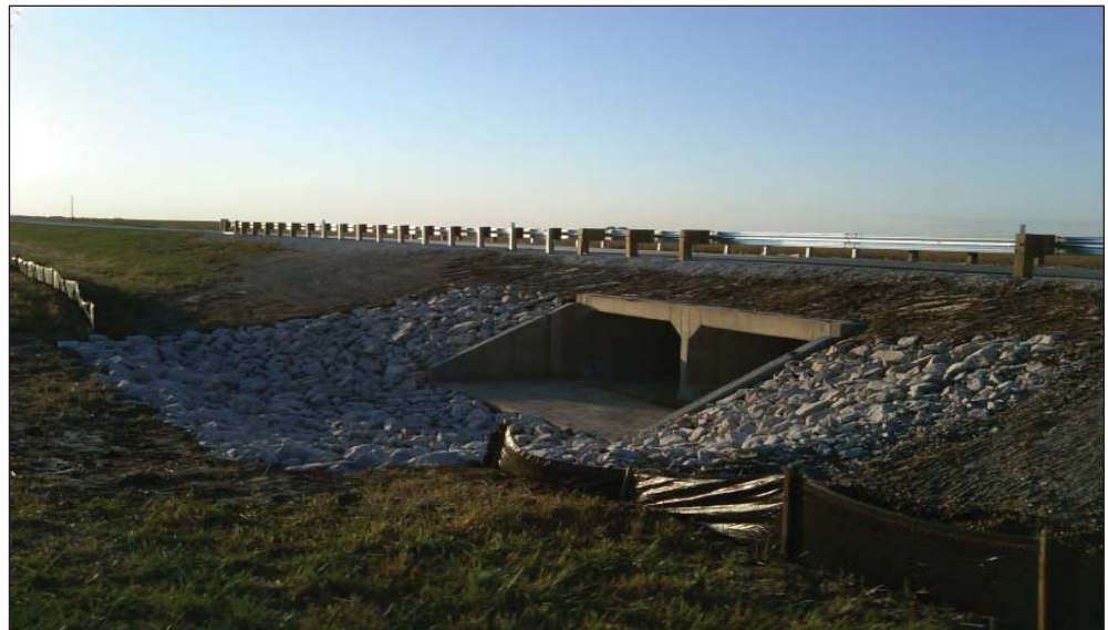
Originally designed as a cast in place box culvert, Bridge B0392 was redesigned as a precast structure to help accelerate the job schedule.
