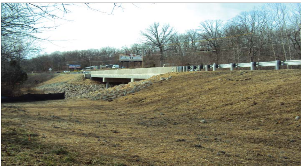
Reconstruction of Bridge B0365 was rescheduled from the summer to fall to avoid inconvenience to tourists traveling to the Lake of the Ozarks and accelerated from 54 days to 42 days to minimize impact to school bus operations.
