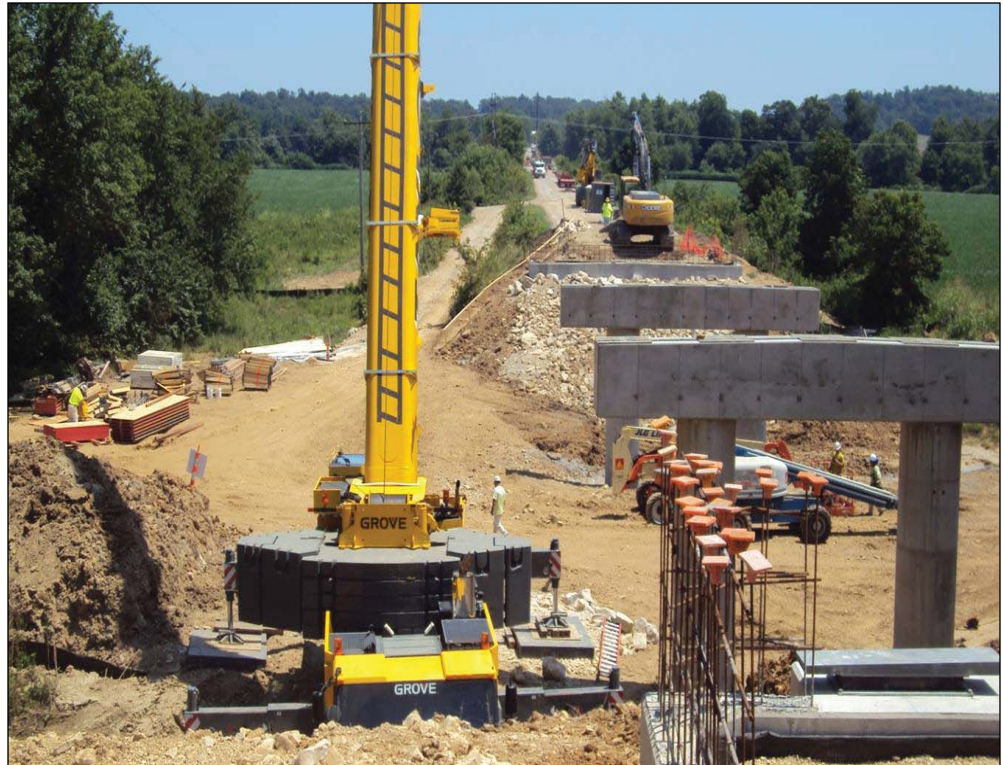
Kozeny-Wagner is ready to set beams on the concrete caps at Bridge B0500.
