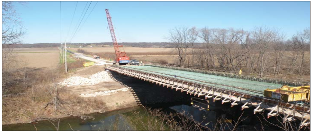
Built by Bleigh Construction, Bridge B0215 in the Northeast Region is a 180-foot long, three span bridge with a concrete deck.
