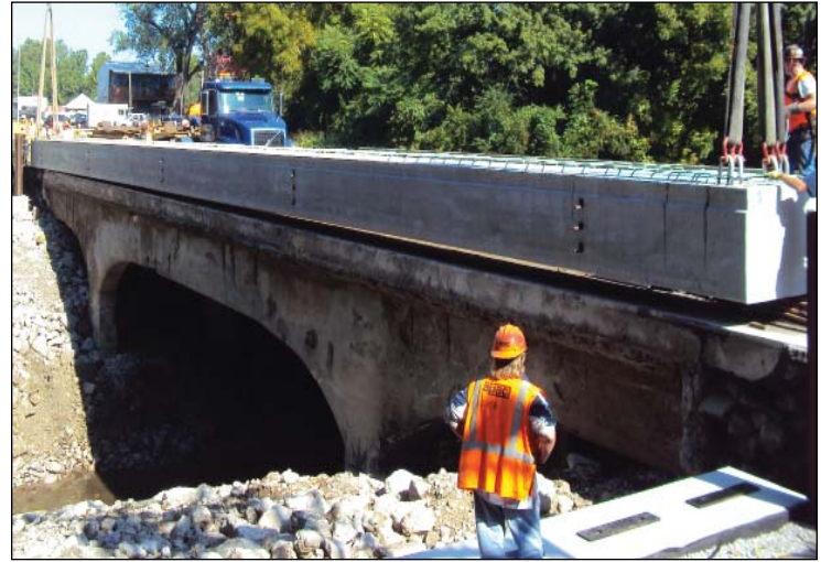
Bridge B0259 was one of 60 bridges completed in the Kansas City region this year, bringing the total number of bridges reconstructed in the region to 91.
