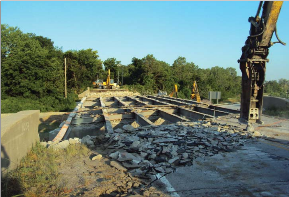
Construction of Bridge B0254, 67th Street over MO Route 350 in Jackson County, is one of the Kansas City Region's more challenging bridges. This bridge spans a heavily traveled route in Raytown and requires full closures of Route 350 during demolition and girder setting activities.
