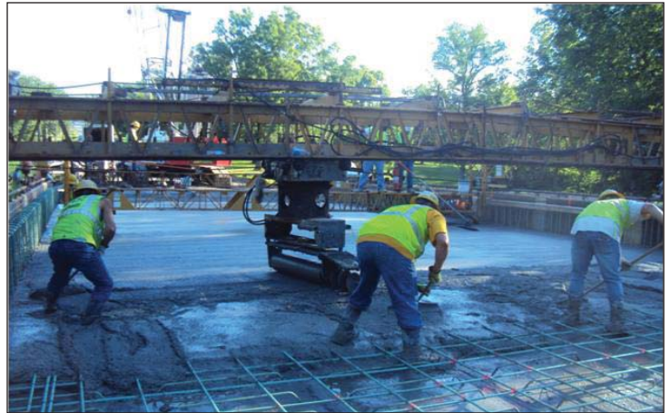
Crews from Clarkson Construction Co. perform the deck pour on Bridge B0057 in the Norwest Region.
