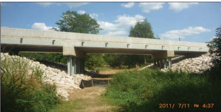
When the Southwest Region completed Bridge B0420 in Jasper County on July 11, construction of the 554 bridges in the design-build program officially reached the halfway point.
